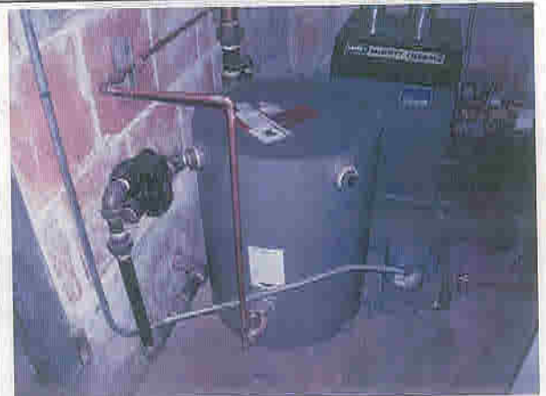
New Condensate-Feedwater Tank
