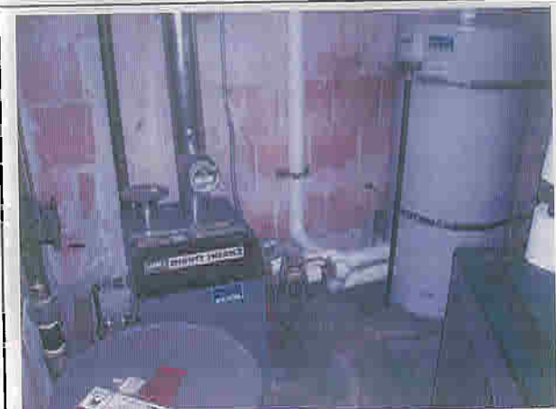
New Domestic Hot Water Boiler & Storage Tank
