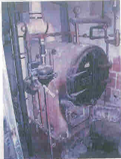
Old Firebox Low Pressure Steam Boiler 18 Unit Multifamily Property
