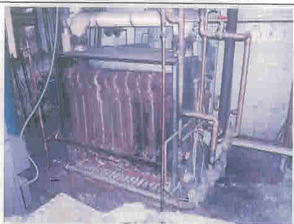
Old Cast Iron Low Pressure Steam Boiler Residential Hotel – Tenderloin Neighborhood
