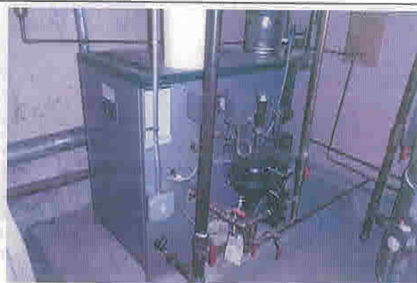
New Low Pressure Steam Boiler 5 Unit Multifamily Property – Richmond District
