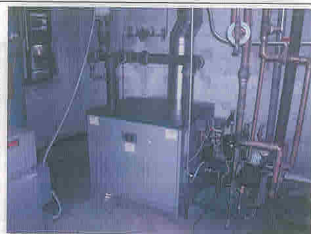
New Low Pressure Steam Boiler Residential Hotel – Tenderloin Neighborhood
