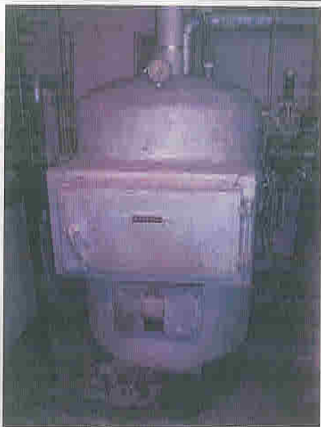
"Old Glory" Low Pressure Steam Boiler 5 Unit Multifamily Property – Richmond District
