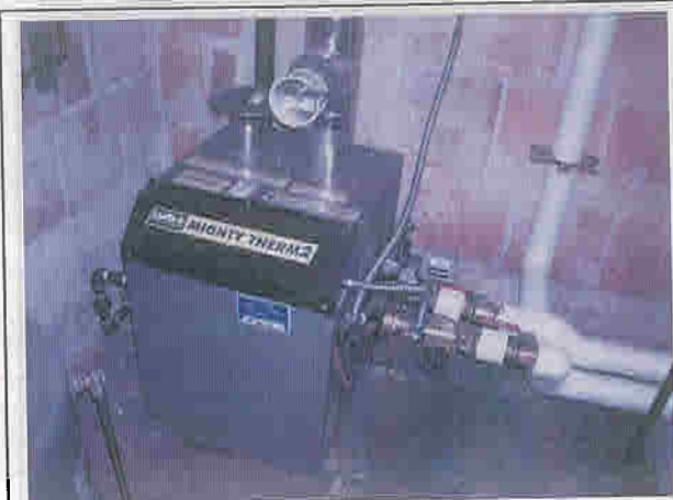
New Domestic Hot Water Boiler
