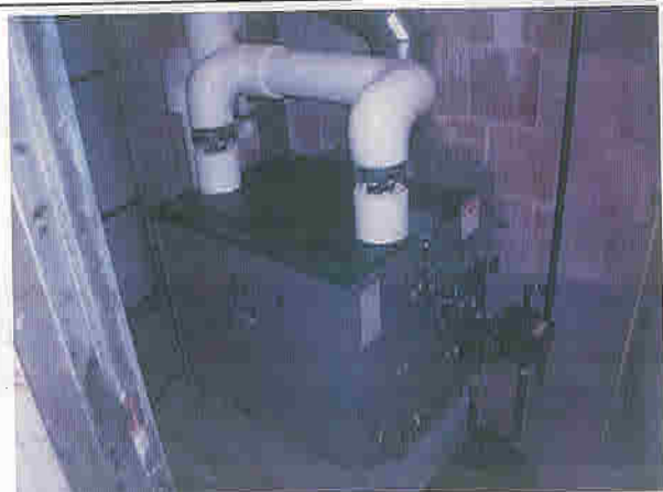
New Low Pressure Steam Boiler
